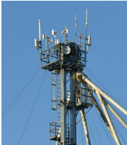
Equipment on Top of Wade Farms Grain
